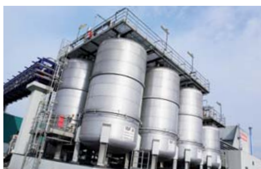
The storage capacity of SAVA is sufficient to ensure five days of operation.
